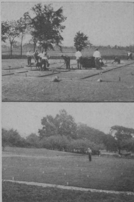
Above, one of the demonstration gardens during construction, and below, how it looks after turf is installed and growing
