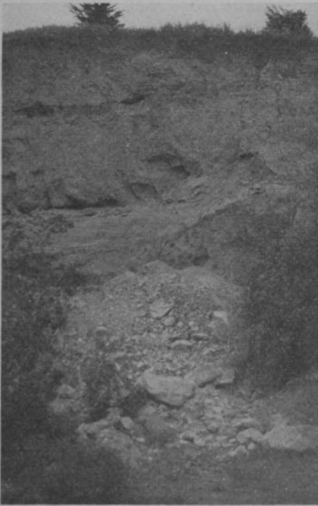
The earthquake shook down this bank at the Virginia Country club.
