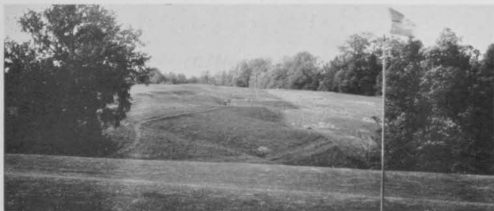
Tees and greens located in the sides of slopes gave Lockwood plenty of drainage problems at French Lick.
