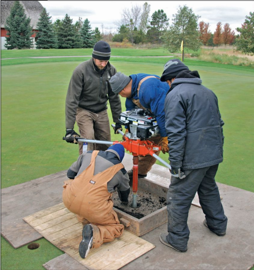
A five-inch auger bit being drilled three feet deep by staff at Medina (Minn.) G&CC to promote water infiltration in swales on native soil greens with no drainage. Channels are back-filled with pea gravel.
