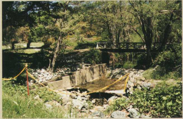
The 1954 fish ladder collapsed under the pressure of torrential rains, combined with river built-up sediments
