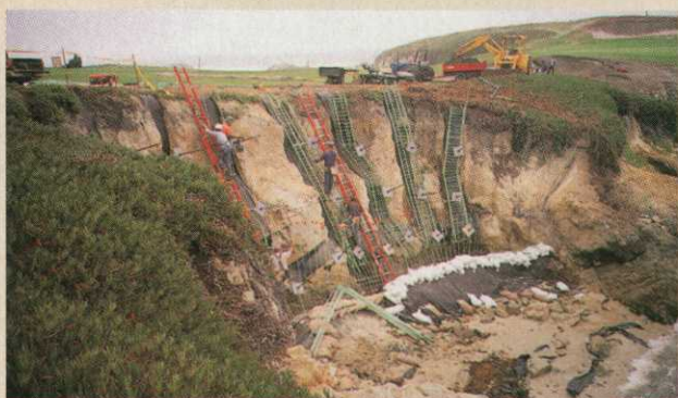
CemRock Landscapes built a steel anchoring system (left) into the side of Cypress Point’s existing shoreline. Then the company built a scaffold-like structure, which provided a frame for the fiber-reinforced concrete.
