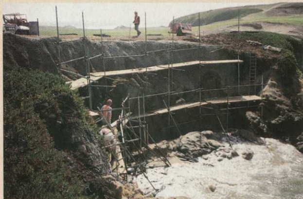
The first layer of 8 inches to 16 inches of structural concrete anchors the structure to the existing seawall.
