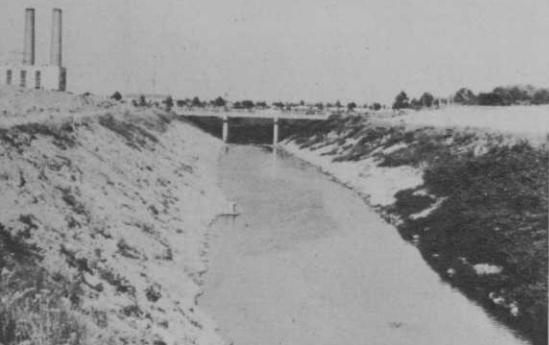
Red Run Drain was enlarged in the mid-1960's due to a growing Southeastern Oakland County population.
