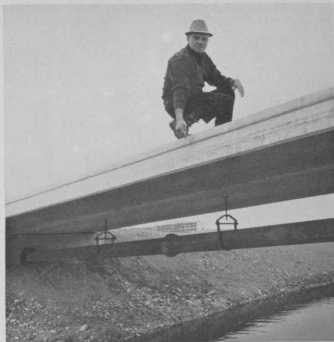
This 8-inch cast iron pipe main supplies all the water for the course. Extending from the pumphouse beyond the bridge, it connects to the 6- and 4-inch cast iron tributaries.
