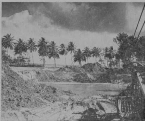
Construction of the 9-hole extension of the 18-hole Dorado Beach GC, Puerto Rico, started last January, will be completed soon. The new 9 begins and ends in the vicinity of the clubhouse.
