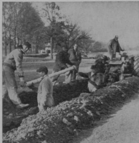
Whitemarsh maintenance crew was able to lay up to 1,000 ft. of pipe in eight hours. Operation went on even during the winter.
