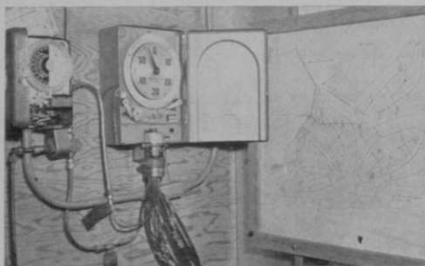
Timing device for control of automatic irrigation system, which is diagrammed on panel at right.
