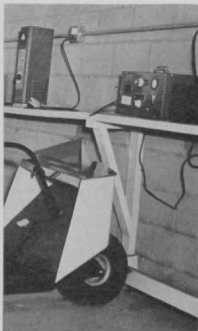
Note charger on counter above car at Olympia Fields CC, Flossmoor, Ill. Diagonal and floor bumpers prevent cars from ramming into walls.
