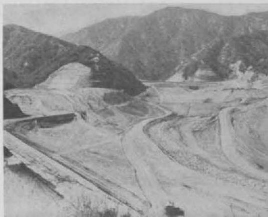
Flood control areas (through center of picture), check dam, (rear), and carved hills mark site of De Bell GC being cut out of Verdugo Hills, Burbank, Calif.
