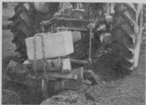
Trench was dug with homemade trencher built on sub-soiler and drawn by a tractor.
