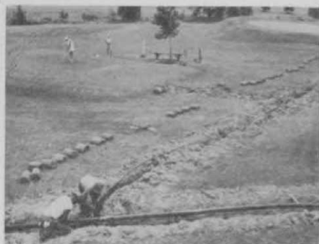
Pipe leading to a green and a tee was installed without interrupting play.
