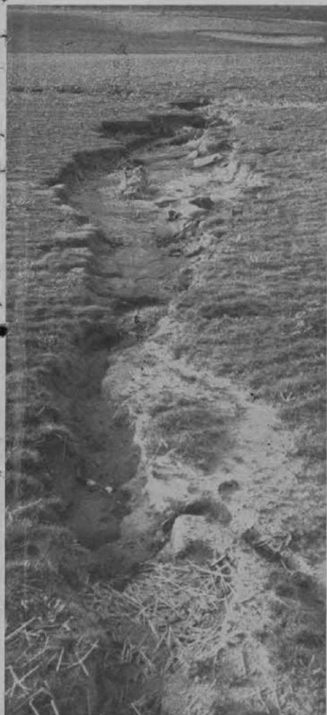
Erosion in untreated soil resulting from heavy rainfall 16 days after seeding. Runoff from 20,000 sq. ft. cut this 18-in. deep trench which is about 3-ft. wide. Ed Knight, author of this article, says his crew had no erosion repair work whatever in areas where soil had been treated with Krilium.
