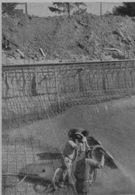
Berkshire CC (Reading, Pa.) pool gets gunite application of concrete under pressure, over heavy steel reinforcing. This provides density and strength. Finished white coat is troweled on by hand after gunite has hardened.
