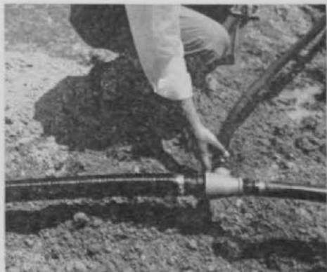
A screwdriver and hack-saw are only tools needed for installation of plastic pipe.
