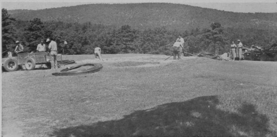
Flexibility of plastic pipe makes installation for watering system comparatively simple operation.
