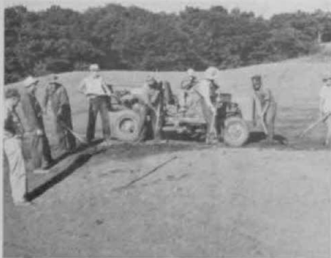
Preparatory to seeding the 4th green at North Oaks workmen rake stones and spread topsoil under the watchful eyes of Bill Fellows, agricultural engineer for Stanley Thompson and Associates, and George Hawkinson, foreman of the construction crew building the course.
