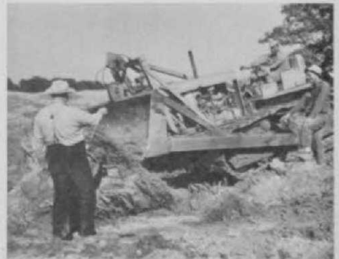
Matt Thompson and Geo. Hawkinson direct removal of a stump by one of the many "cats" which moved the landscape around during the construction of North Oaks Golf Course.
