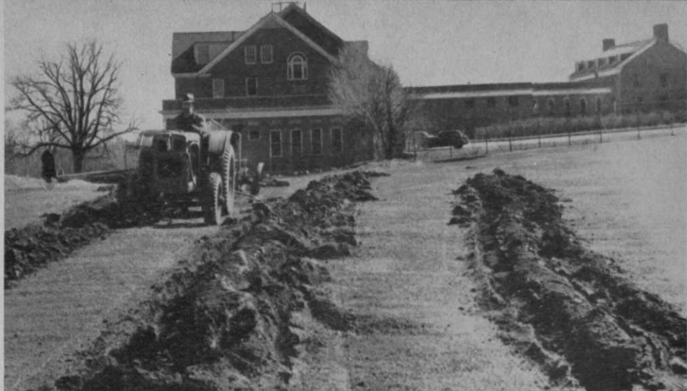
Tractor plowing six acres of property at Wykagyl CC (New Rochelle, N. Y.), for member V-gardens. By April 1, over 50 families had reserved plots, some as large as 10,000 sq. ft., under the strict requirement that all plots neglected by the members will be maintained by the club and the cost assessed against the members. (N. Y. Times Photo).
