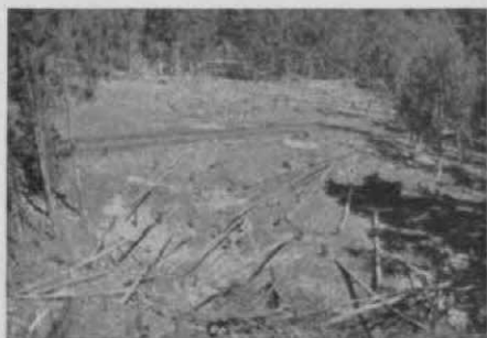
An idea of how much clearing was needed is given in this view of the practice fairway.
