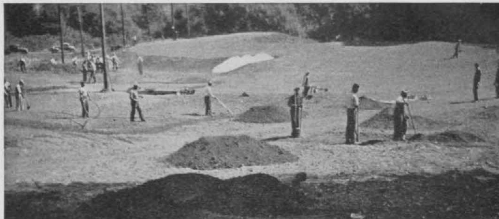
Construction view at Tilden Park. Workmen are seeding the 4th green in the background, while others nearer the camera are spreading topsoil for the fairway.
