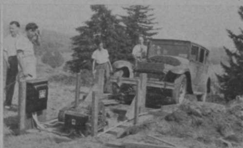
Hoist and controls at upper end of tramway. After photo was taken, this machinery was enclosed from the weather.
