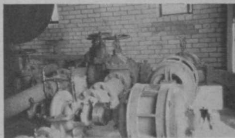
View of main pump-house at the Country Club, Brookline.
