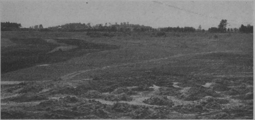
Topsoil on No. 9 green at Portland (Me.) municipal course before spreading. No. 1 fairway at left being disced
