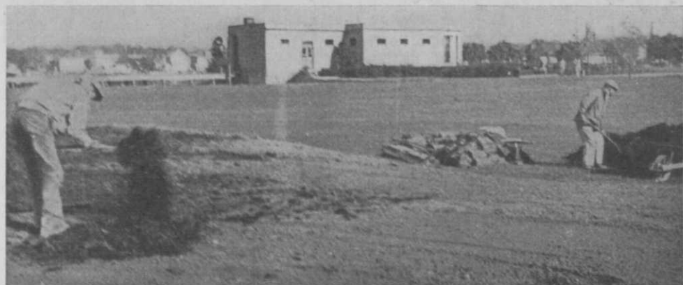
Rebuilding a green. The turf has been removed and will be replaced after defective contours have been corrected and the workmen finish applying well-rotted manure to the area.
