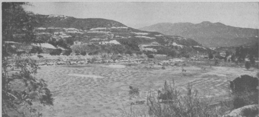
A new 9-hole golf course is being built in this old river bed at Pasadena. The piles are topsoil to cover the sandy bottom
