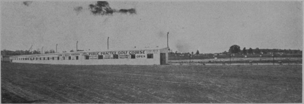
A driving range lighting installation showing 500-watt floodlights installed on shelter.
