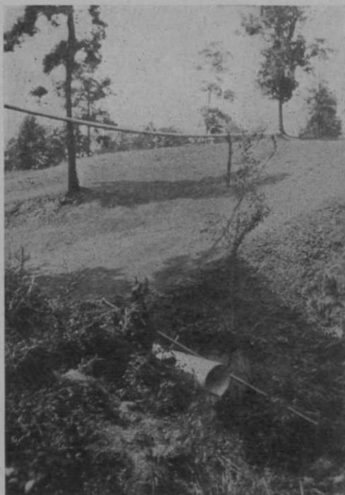
Installation at lower side of fairway No. 8 which stopped undermining of a bulkhead at this point.
