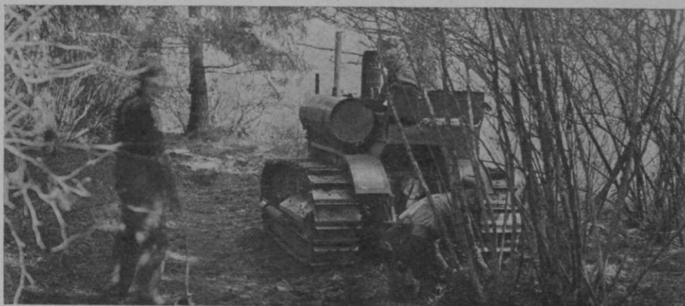
During construction of the new Evergreen Golf Course (Vancouver, Wash.), a Caterpillar 30 tractor made short work of the land clearing
