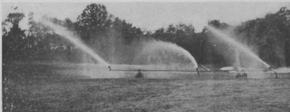
This makeshift fairway watering outfit at Glen Oaks is one of the drought desperation measures that the on-rush of fairway watering installations will eliminate.
