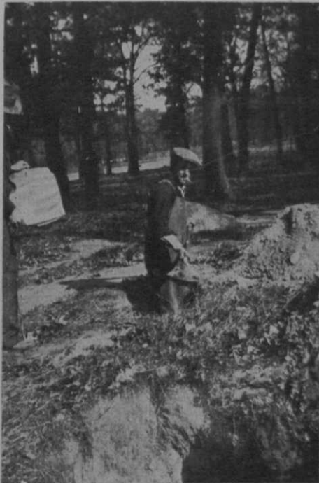
Hunting for pipe connections. This expensive work shows value of accurate map,
