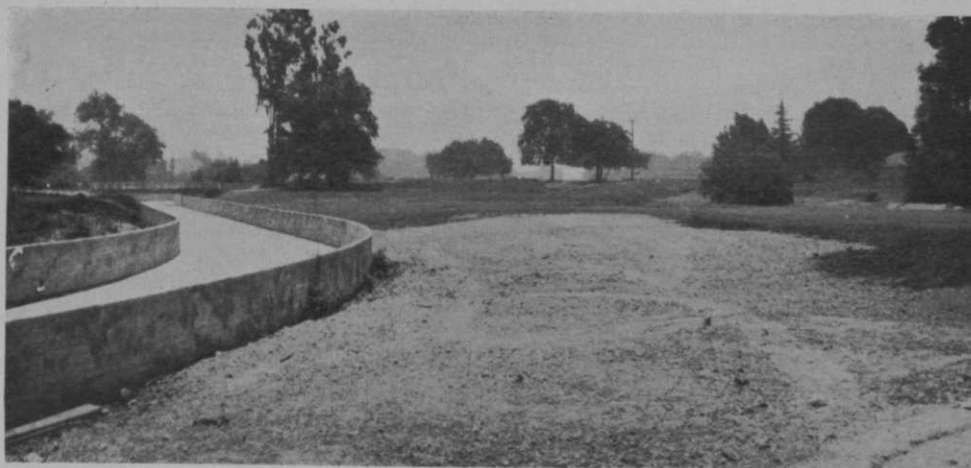
To prevent fairway erosion during the annual rainy season, this concrete flume has been built at the San Gabriel (Cal.) C. C. in the former river-bed. This view was taken during construction of the flume.
