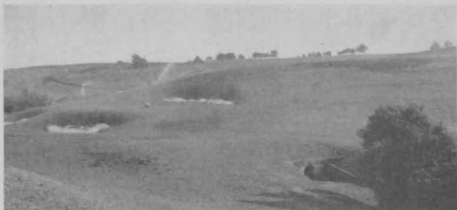
Restored green on the Los Angeles Country Club course after installation of new storm drain.
