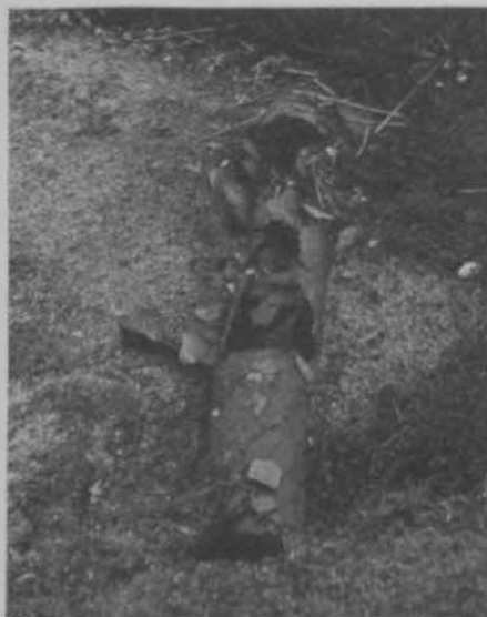
They put two drain-tiles, one inside the other, in this installation; but it didn't handle the strain.
