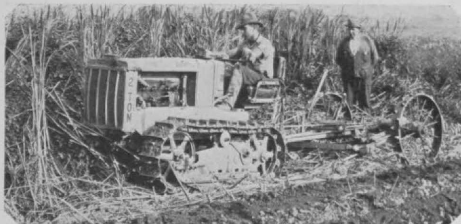
Plenty of clearing was necessary during the construction of the Sandy Beach (Ohio) course, but utilization of modern, cost-cutting machinery such as the Caterpillar tractor shown here, resulted in a job of record speed and thrift.
