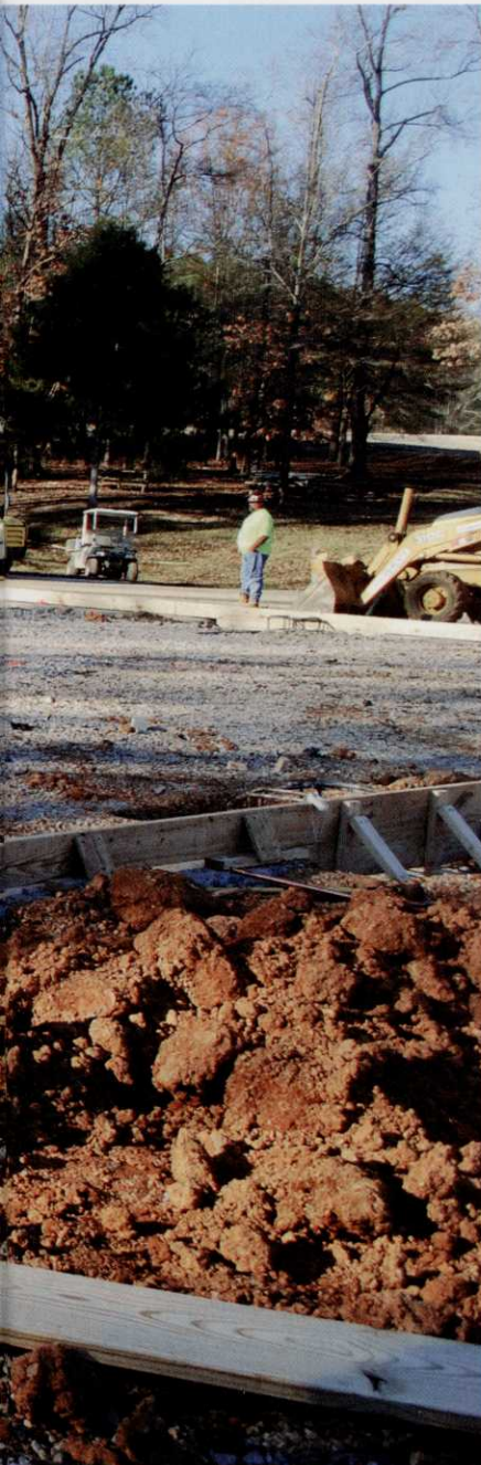
Construction of the new maintenance facility at FarmLinks Golf Club at Pursell Farms in Sylacauga, Ala.
