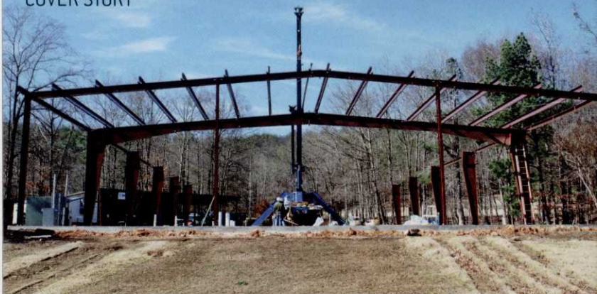
The frame of the new maintenance facility as it was under construction.
