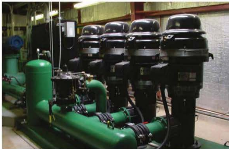
Scheduling your pump system operation is a way to help reduce energy and maintenance costs.
