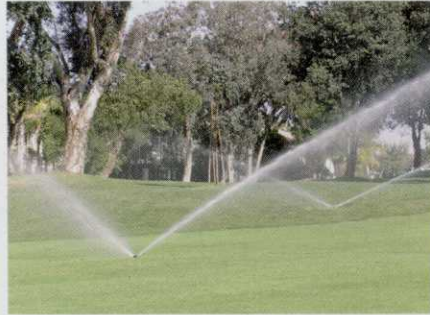
Profile retrofit nozzles have tiny notches pressed into the nozzle face along the stainless steel insert. The notches strip away a small amount of water from the main stream, dropping it closer to the sprinkler head, spreading the stream more uniformly.
