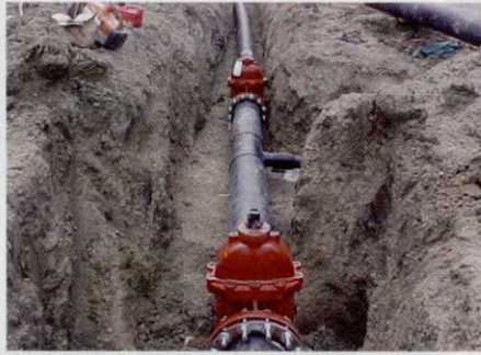
An assembled mainline gate valve.
