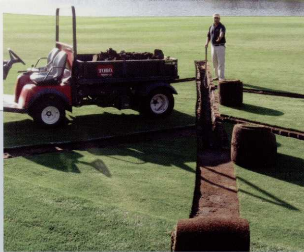
The Ridge at Castle Pines has installed more than a mile of drainage to mitigate high sodium since 2004. Photo: David Soltvedt
