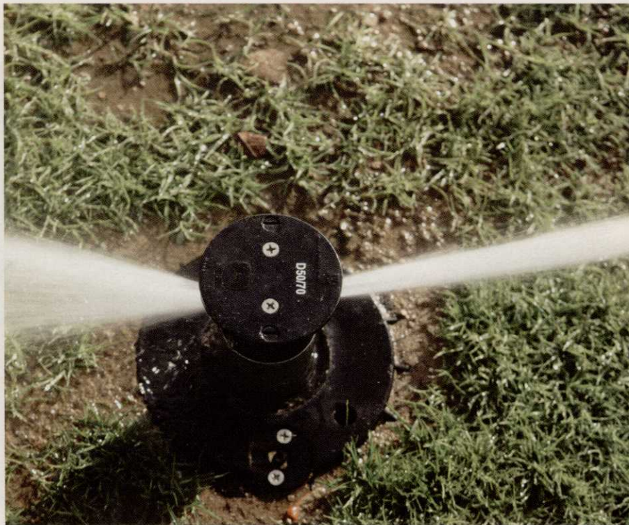
The number of irrigation heads was increased because of the windy site. Photo: EPIC Creative
