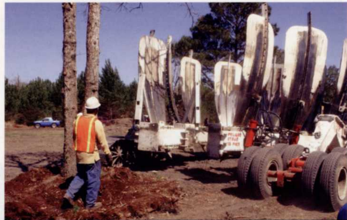
The Daniel Island Co. hired Tree Doctor to minimize the number of trees that are removed or damaged during course construction.
