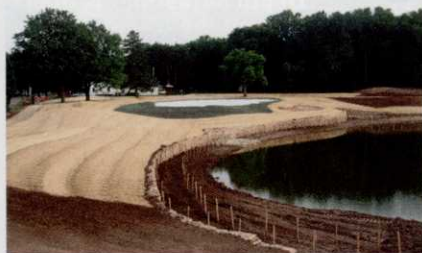
The third hole at Reid GC. Top left: Grassing. Bottom left: Shaping and earthwork. Right: Grow-in from the tee.
