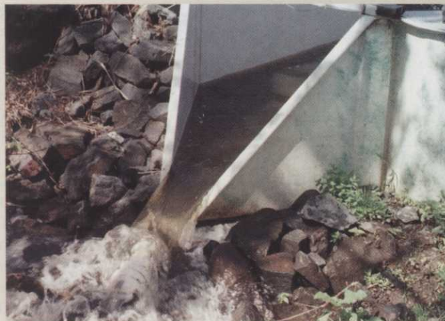
Figure 2. Installed H-flume at Northland Country Club (NCC) in Duluth, MN.
