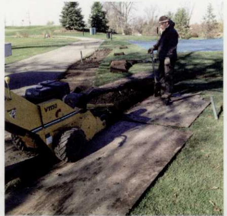
Corrugated drain lines with pea gravel were installed to move water from the tee surface.
