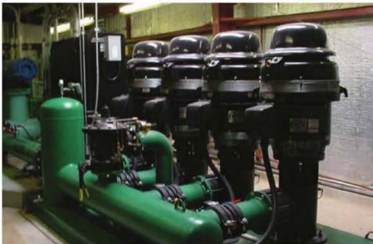
Scheduling your pump system operation is a way to help reduce energy and maintenance costs.
