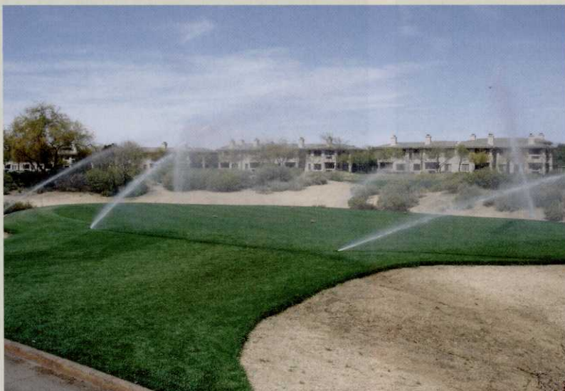
Many courses need to replace their whole irrigation system, not just parts.
