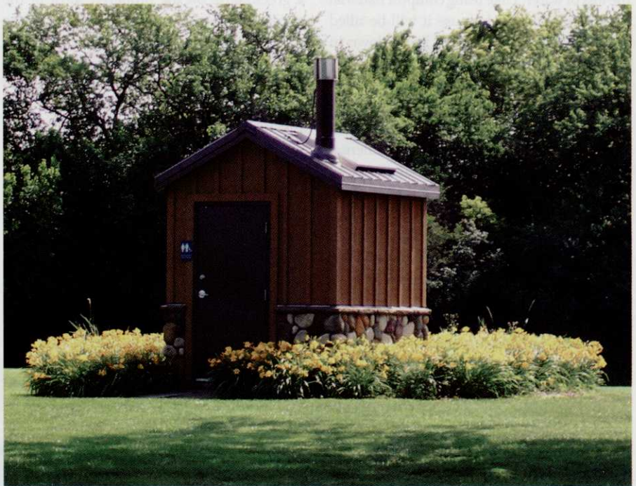
The Biological Mediation Systems facility composts without water or electricity and operates a ventilation fan via a solar power unit on the roof.
