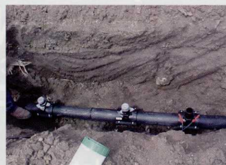
An electro-fused 4-inch by 2-inch saddle.
